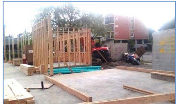
Construction at Salvation Army, Renton. This photo [dated 05/24] shows the extensive amount of construction at the site. (Photo by Dave Smith KB7PSN).
