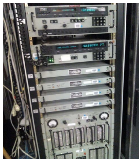
Photo: 1-KW HF Transmitter [Article-(Table)-Continued on Page 6]
